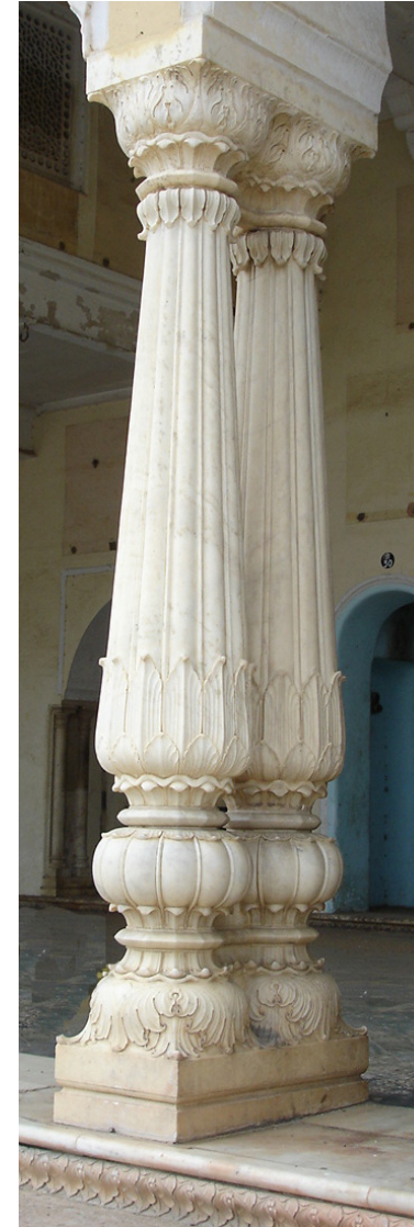
3. Column detail from Swinton Jacob's building inspired from existing architectural details in Jeypore and Amber.-
